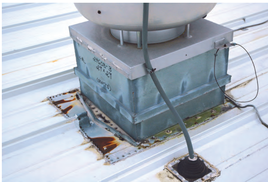
Rust can develop when roof accessories, like curbs or flashings, use a lower-grade coating than the roof panels around them. Here, the roof is holding up well, but the curb is not. PHOTOS COURTESY OF S-5! AND THE METAL ROOF ADVISORY GROUP, LTD.
