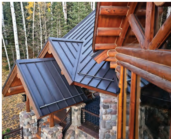
The Yellow Brick Road log cabin in Colorado features a standing seam metal roof with S-5! ColorGard 2.0 snow retention to reduce the risk of rooftop avalanches. PHOTO COURTESY OF ROOFING CONTRACTOR WHITE CASTLE ROOFING.
