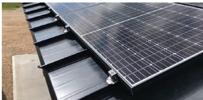
The solar array on this barn in British Columbia, Canada, is mounted using the S-5! PVKIT rail-less solar mounting solution for metal roofs, where the standing seams of the roof act as built-in rails. PHOTO COURTESY OF S-5!
