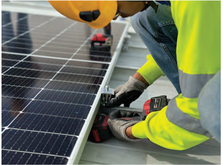
Installing solar panels with penetration-free attachment solutions preserves the integrity of a standing seam metal roof while simplifying the installation process. PHOTO COURTESY OF S-51
