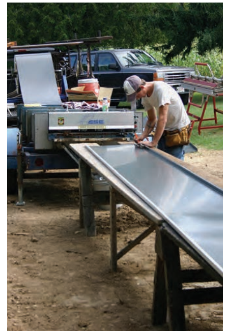
Jason Golke marks the panel where it has to be cut and folded before it is installed.
