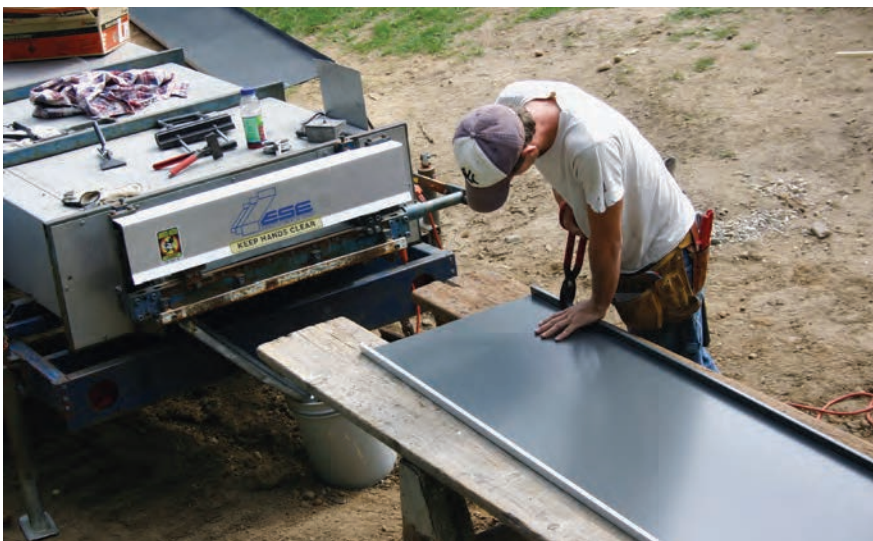
Jason Golke is a third-generation metal roofer, working with his father at Jim’s Roofing Service & Son of Waupaca, Wis. He operates the roll former and helps install the double lock mechanically seamed panels.
