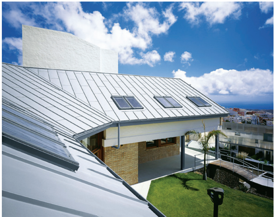
This private residence, Montana del Socorro , is located in Tafira Baja, Spain. The roof is 250 square meters of RHEINZINK's pre-weathered blue-grey angled standing seam. Architect Samuel Steiger Ritvo of Las Palmas Gran Canaria, Spain was in charge of design. RHEINZINK PHOTO
