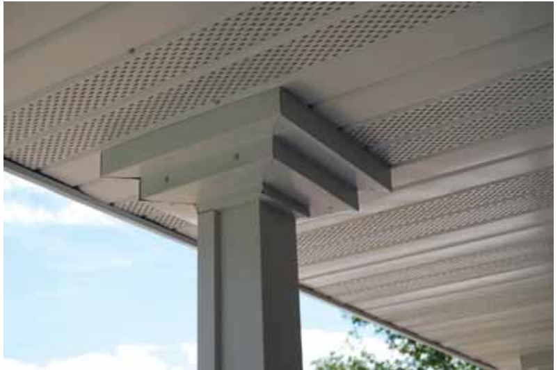
Vented soffit. Air inlet volume should match air exhaust volume. COURTESY OF MWI COMPONENTS.
