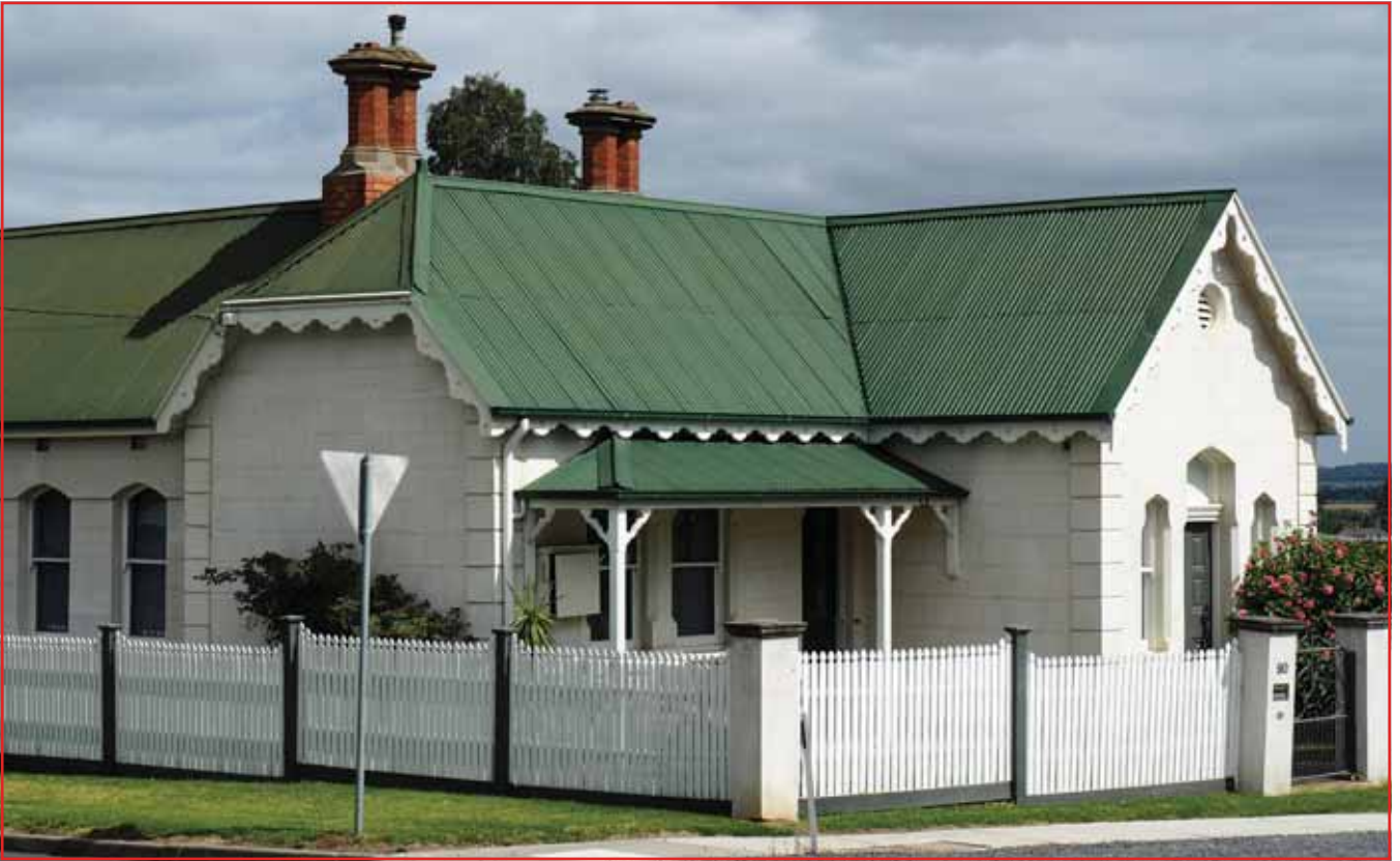
Corrugated residential roof installed 75 years ago in Australia. PHOTO COURTESY OF APPLICAD, AUSTRALIA
