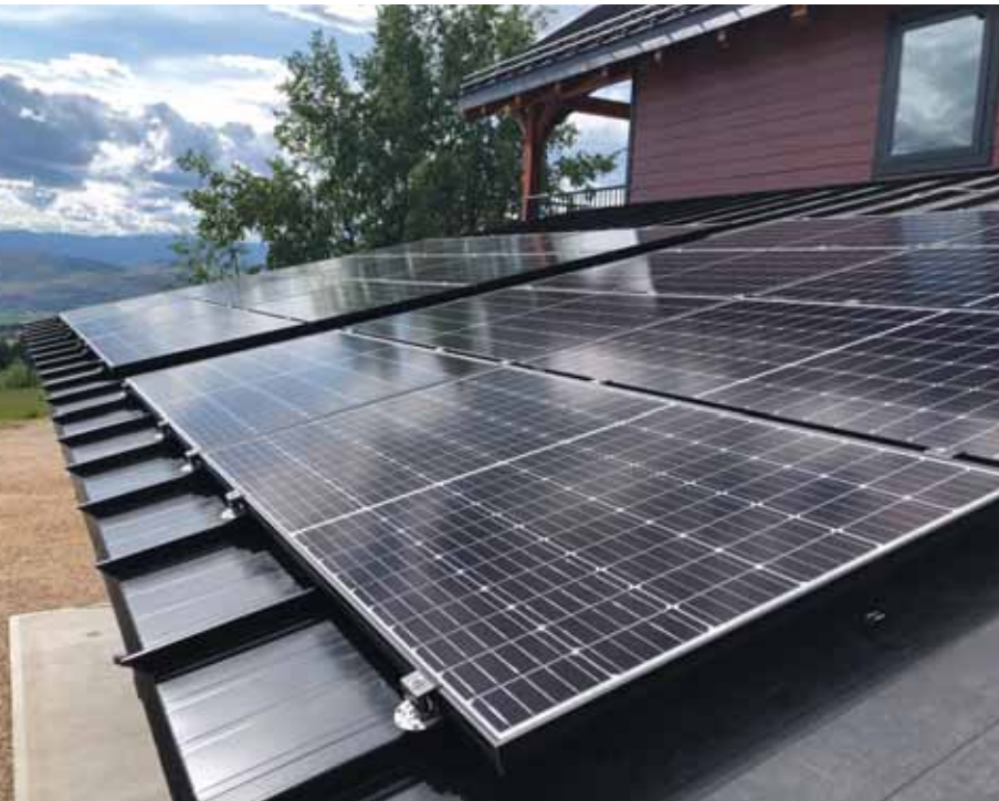
Solar system installed with an S-5! PVKIT™
