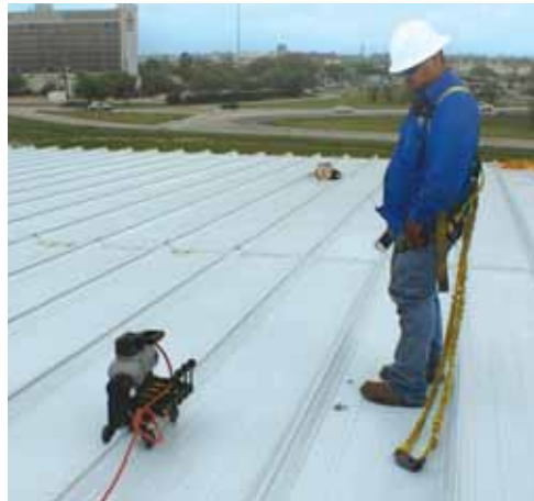
Keeping a watchful eye on the seamer will quickly catch problems that arise. PHOTO COURTESY OF DI ROOF SEAMERS.
