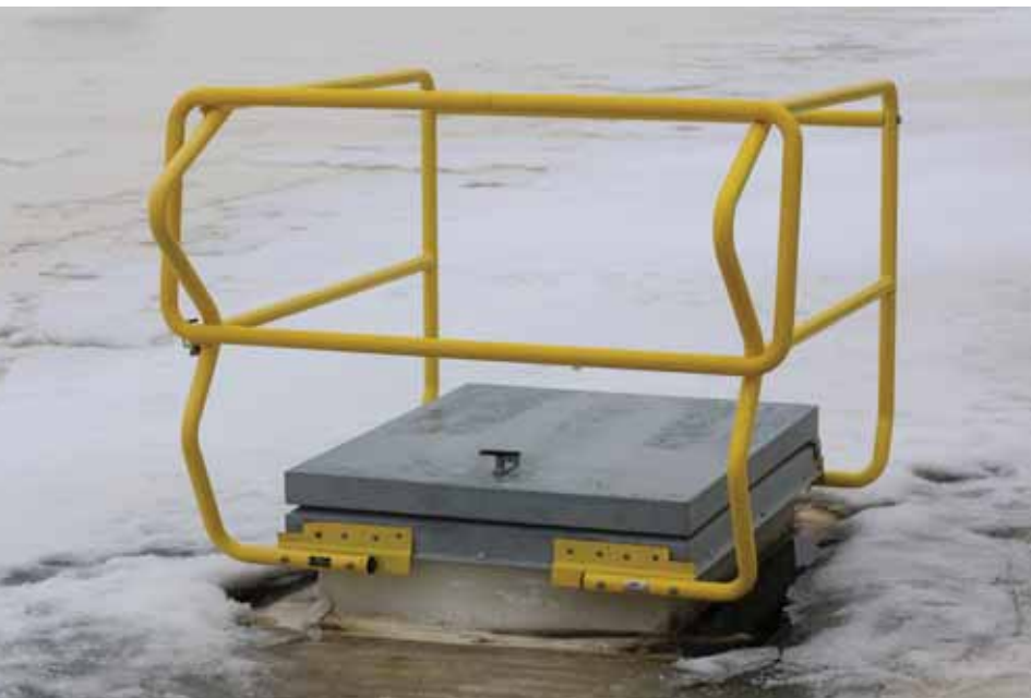
Roof hatch doors can become hazards during windy conditions. Photos courtesy of Diversified Fall Protection.
