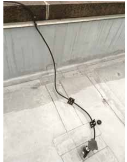
This lightning protection system was apparently "re-installed" after some roofing work, but it was not installed correctly as the cables are not fastened to the roof and the air terminals are incorrectly located.
