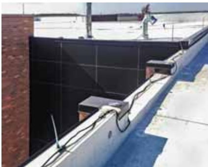
Re-installing a lightning protection system requires special attention and the knowledge of a certified installer. After completing some roofing work on this project, this system is reinstalled correctly: the conductors are straight, no sharp bends in the coil and it's fastened correctly.
