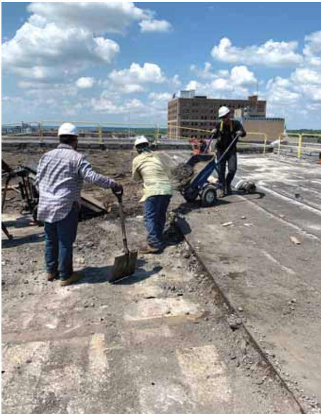
Western Specialty Contractors workers installing new Hydropack roof garden system. Photo courtesy of Western Specialty Contractors.
