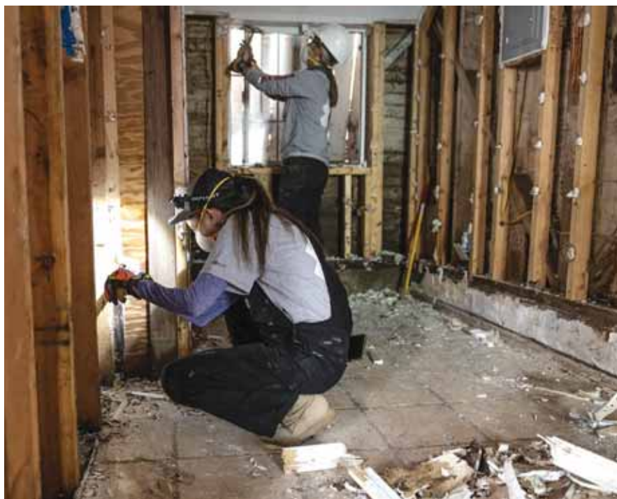
Flooding response in San Diego. PHOTOS COURTESY OF TEAM RUBICON.
