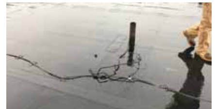
All sorts of problems become possible when lightning protection cables are not properly fastened.
