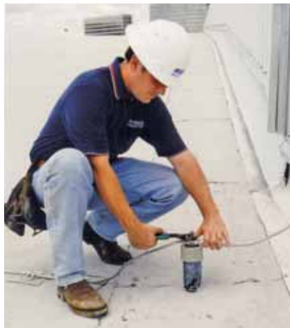
An installer correctly connects and fastens a lightning protection system in this through-roof application.
