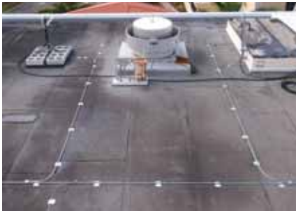
A neatly installed, standard-compliant lightning protection system roof network.
