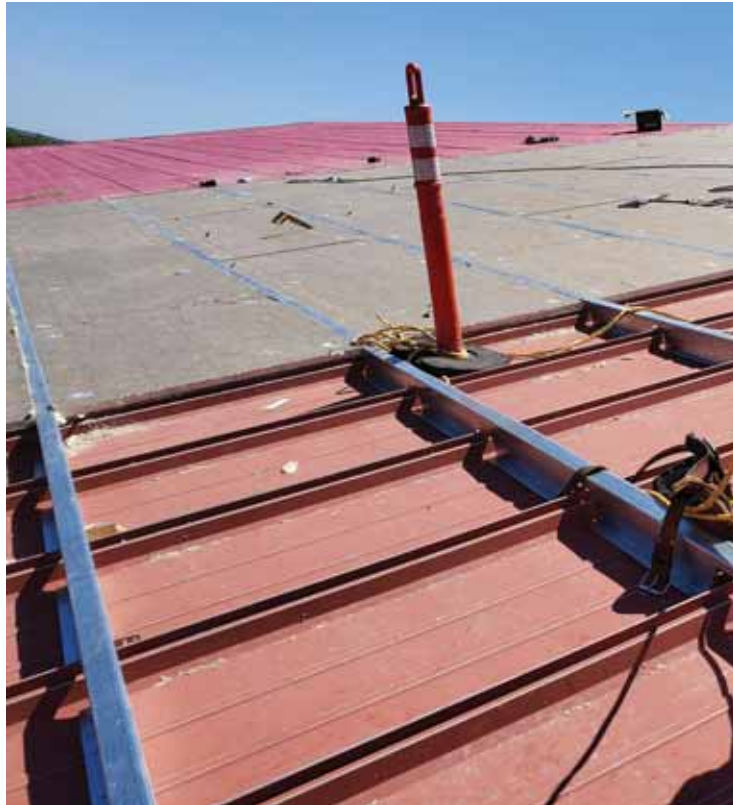
Rigid insulation panels are added on top of the old standing seam deck.
