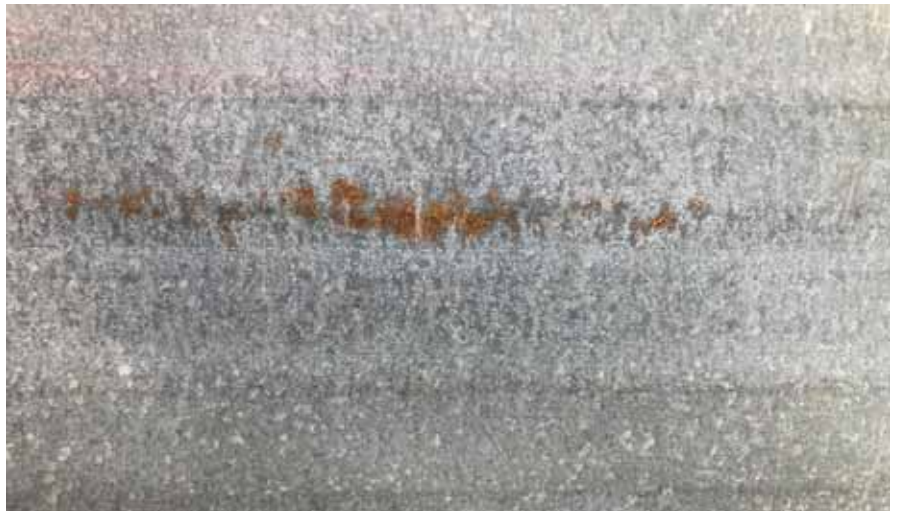
Galvanized steel exhibiting rust.
