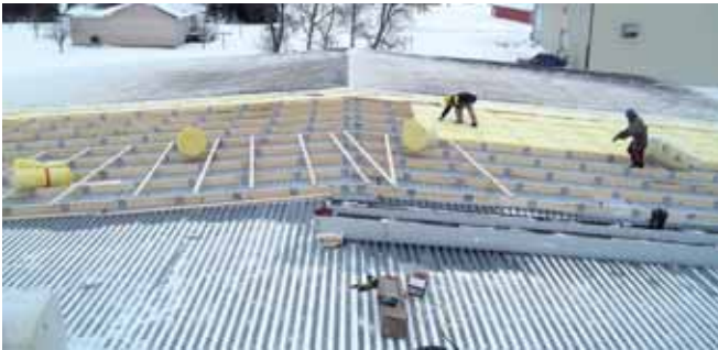
A school roofed with Q deck gets an upgrade using the 2 x 8 retrofit clip with a 2” trapezoid thermal block system. PHOTOS COURTESY OF RETROFIT CLIP
