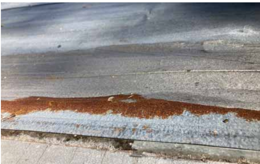
Rusting galvanized steel where stressed.
