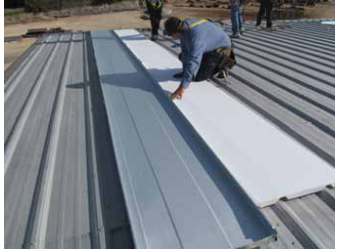
A molded insulation panel is layered on top of the old through-fastened roof deck before it is re-covered. PHOTO COURTESY OF MCELROY METAL.
