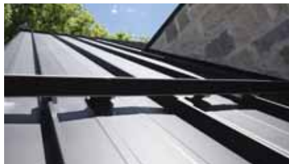
S-5! ColorGuard snow retention. PHOTO COURTESY OF S-5!
