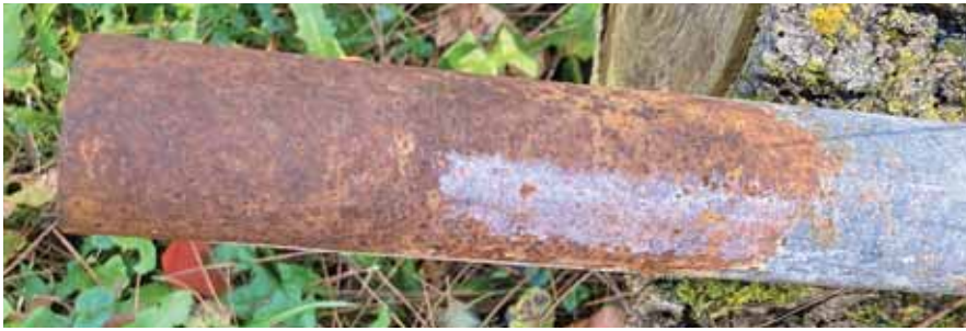
Galvanized pipe with soil exposure.
