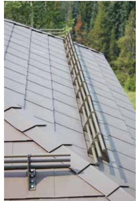
Snow fence installed on a metal shake roof. COURTESY OF ROCKY MOUNTAIN SNOW GUARDS
