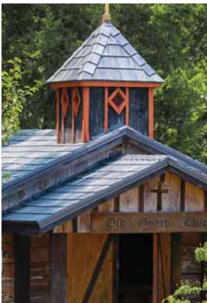
Smith Roofing & Exteriors worked with Kingston, Tennessee, and True Metal Supply to authentically replicate roofing on historic buildings at Fort Southwest Point. (Kasselwood Metal Shingles from True Metal Supply.) PHOTO COURTESY OF SMITH ROOFING & EXTERIORS.
