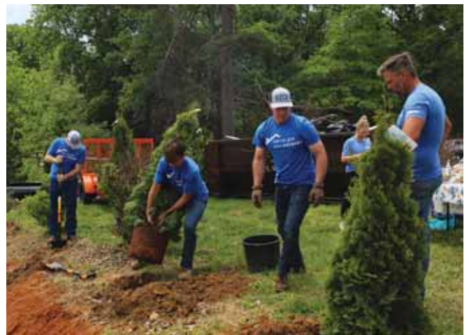
A crew from FLOW Roofing and True Metal Supply also worked together to rebuild the carport and landscape the property.
