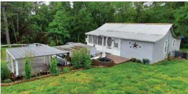
Before: Leaky roof needed replacement. PHOTOS COURTESY OF FLOW ROOFING AND TRUE METAL SUPPLY.
