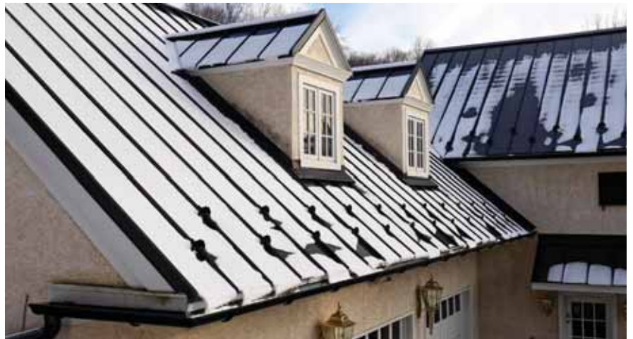
Snow guards are attached to the standing seams on these roofs. PHOTO COURTESY LEVI'S BUILDING COMPONENTS
