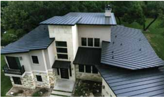
APEX Roofing of Georgetown, Texas, was able to complete the job in just four days, overcoming challenges presented by the low slope of the roof by adding winter guard underlayment. PHOTO COURTESY APEX ROOFING/MRA
