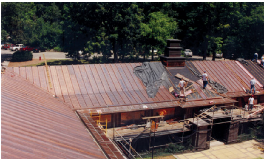
NIKO Contracting replaced the traditional batten seam copper roofing, built-in copper gutters, flat lock copper eave covers with faux standing seams, and decorative copper soffit at the Kingswood School at the Cranbrook Educational Community in Bloomfield Hills, Mich.
