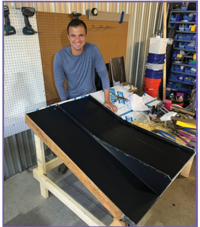
Individual advanced 24-gauge painted steel detail training in Reading, Pennsylvania. PHOTOS COURTESY OF JOHN SHERIDAN, SHERIDAN TOOLS.
