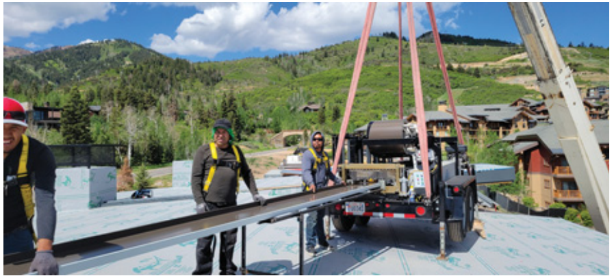
The roll-forming trailer is jacked and stabilized to hover just over the roof so as to not put extra weight on the roof structure. PHOTO COURTESY OF SALTEDMETALS ARCHITECTURAL METALS DESIGN AND CONSULTING
