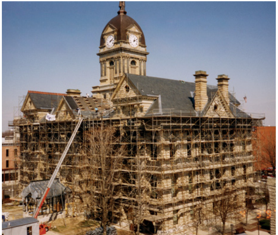
NIKO Contracting handled the entire exterior restoration at the Hancock County Courthouse in Findlay, Ohio. The project included a new copper dome, refurbishing the sheet copper statues, new lead-coated copper gutters and flashing, new lead-coated copper standing seam roof, slate with lead-coated copper snow guards fabricated by NIKO, new roof decking, new historic wood windows and doors, and masonry restoration. NIKO CONTRACTING PHOTOS
