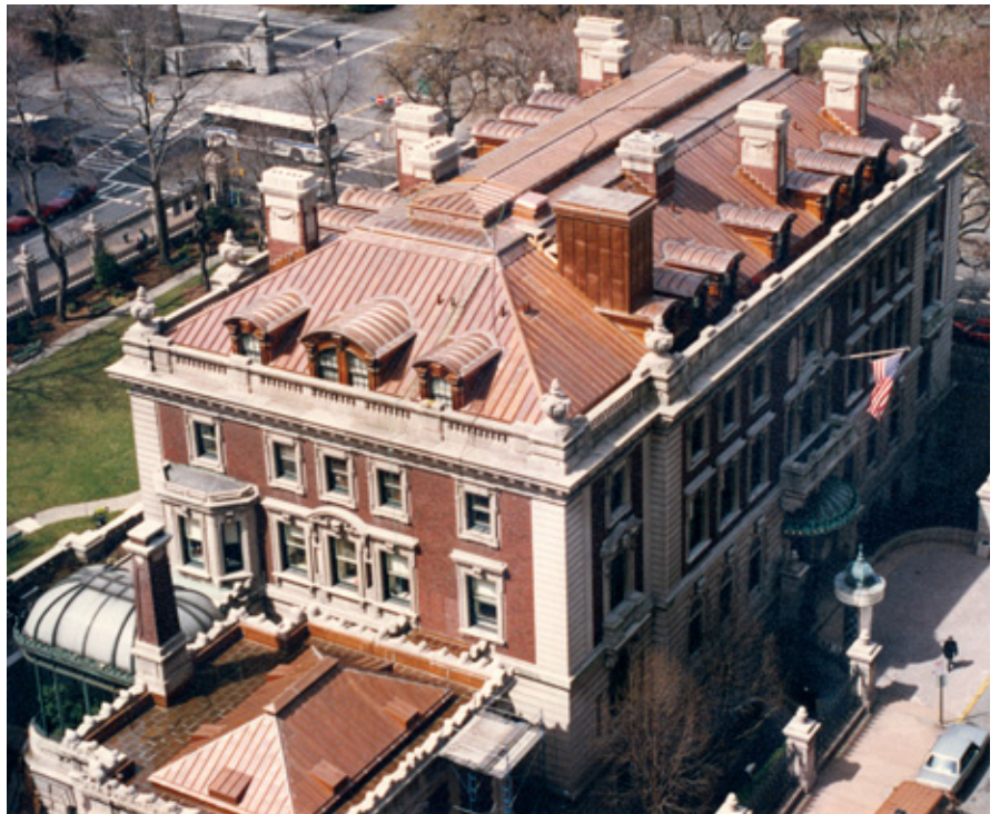
The Cooper-Hewitt National Design Museum in New York City was a project that kept NIKO Contracting busy for almost two years. NIKO replaced all the copper roofing gutters and ornamental copper, along with the wood and concrete decking.
