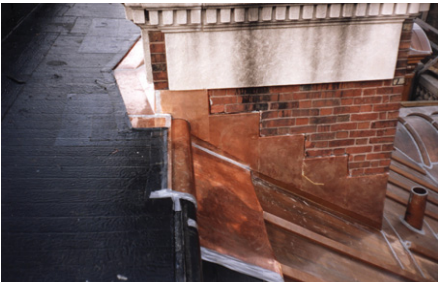
A closer look at the copper batten seam roofing and copper flashing of the chimney during the roof restoration of the Cooper-Hewitt National Design Museum in New York City.
