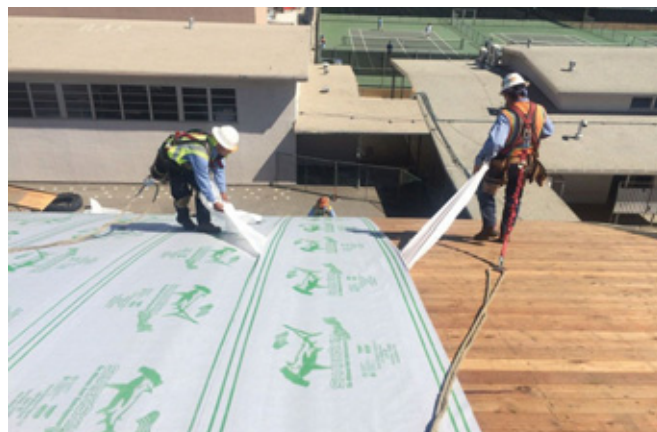
SharkSkin self-adhesive underlayment applied to the deck of Newbury Park High School. PHOTO COURTESY OF SHARKSKIN/KIRSCH BUILDING PRODUCTS.
