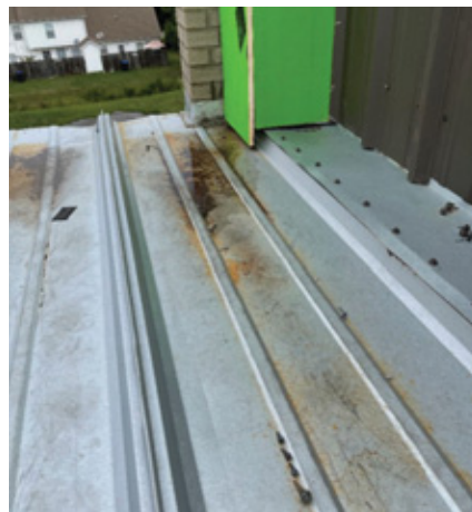
These installation errors occurred when the brick mason scratched and bent the panel downward creating a ponding condition. The panel does not have enough slope to shed the water. Also, screws were left on the roof, which created a rusting problem. PHOTO COURTESY OF STRUKTUREONE GROUP.
