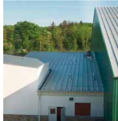
While roof loads are usually lower than ground loads, aerodynamic shade (drift load, shadow load) can cause roof design loads to be several times that of ground snow.
