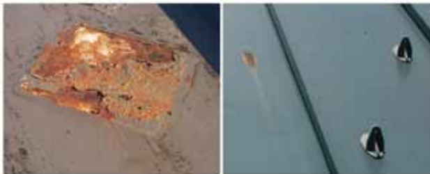
The adhesive bond is to paint. If the adhesive does not fail, the paint may fail, leading to corrosion.
