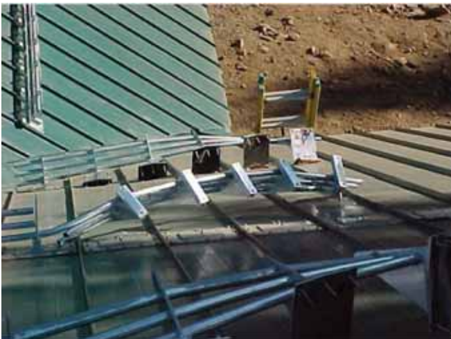
Mechanical bracket attachment (for face-fastened roofs only) can also work successfully when tested and engineered correctly. This one wasn't.
