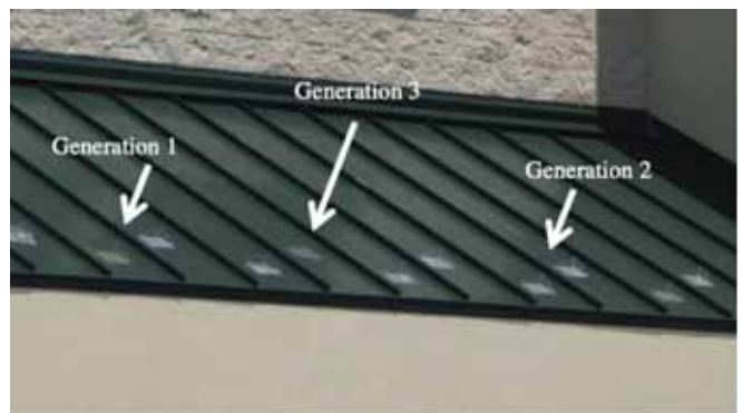
Adhesive holding capacity diminishes over time when exposed. There are three generations seen on this 8-year-old roof.
